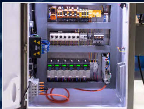
2. System Control Panel
